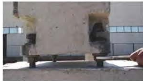
All the concrete elements are joined by bolted steel connections, all reversible reusable in the future.
